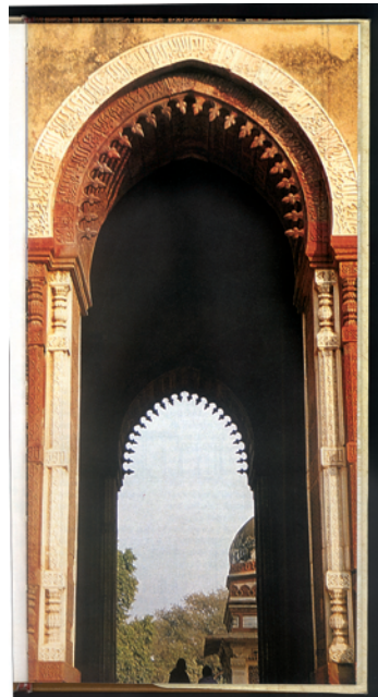
Fig: 22.5a A 'true' arch. The 'keystone' at the centre of the arch transferred the weight of the superstructure to the base of the arch.
